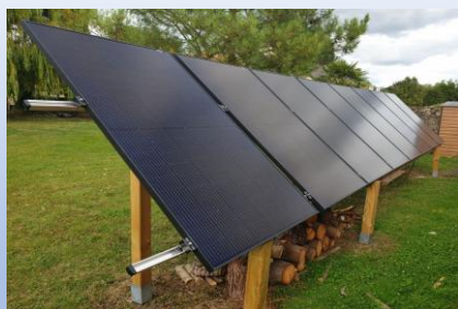
Auto – Installation 3 kWc
